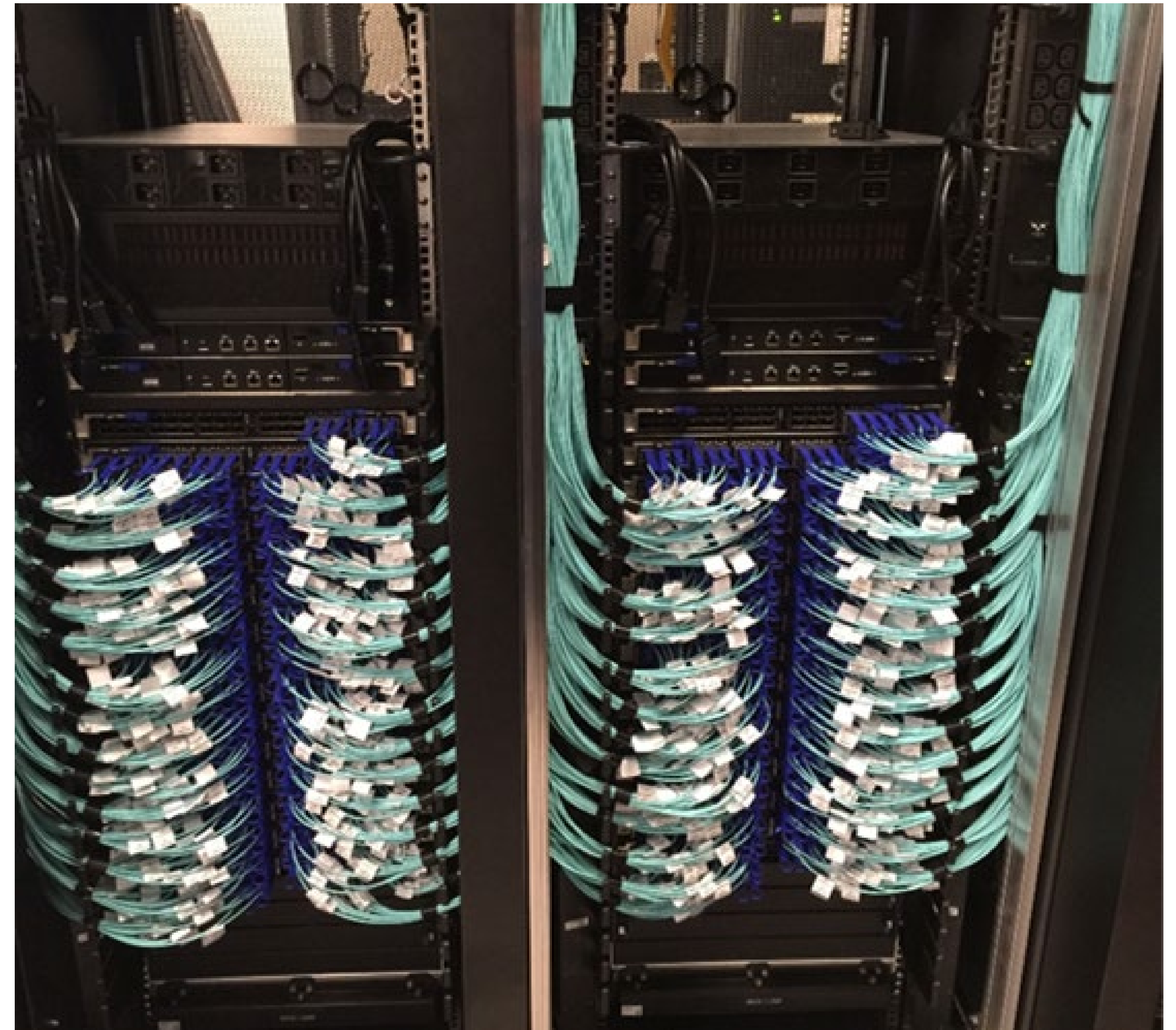
Example of proper cable management
