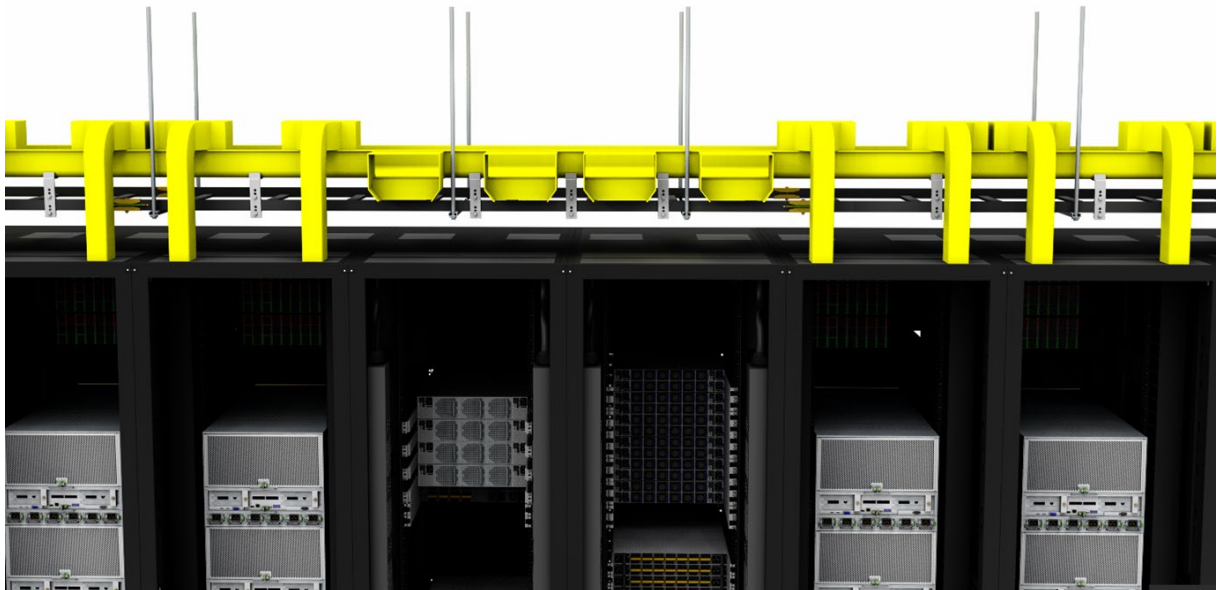
Figure 19. Typical overhead cable management detail—rear
