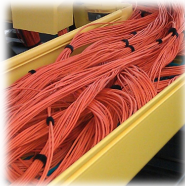
Figure 32. Cleanly deployed cables
